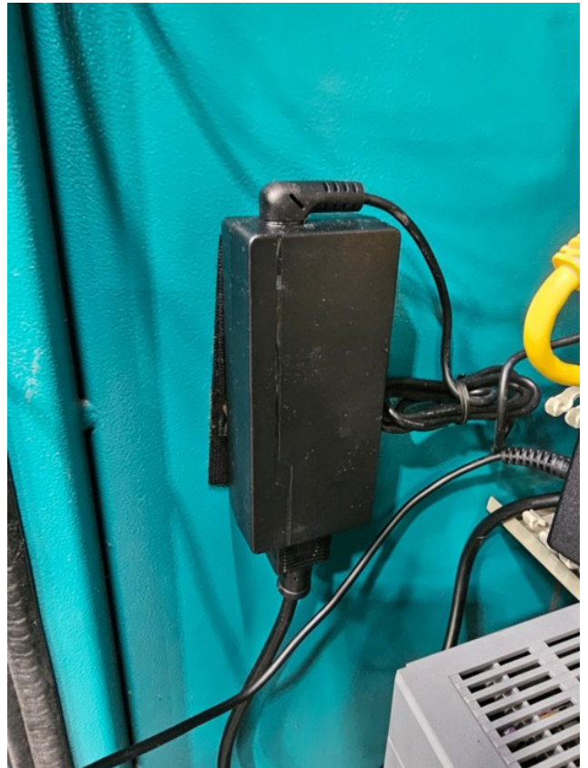
Inspection PC Power Supply
